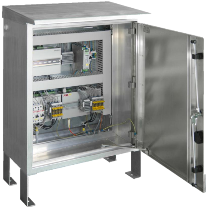
Outdoor cubicle with SAM600 system
